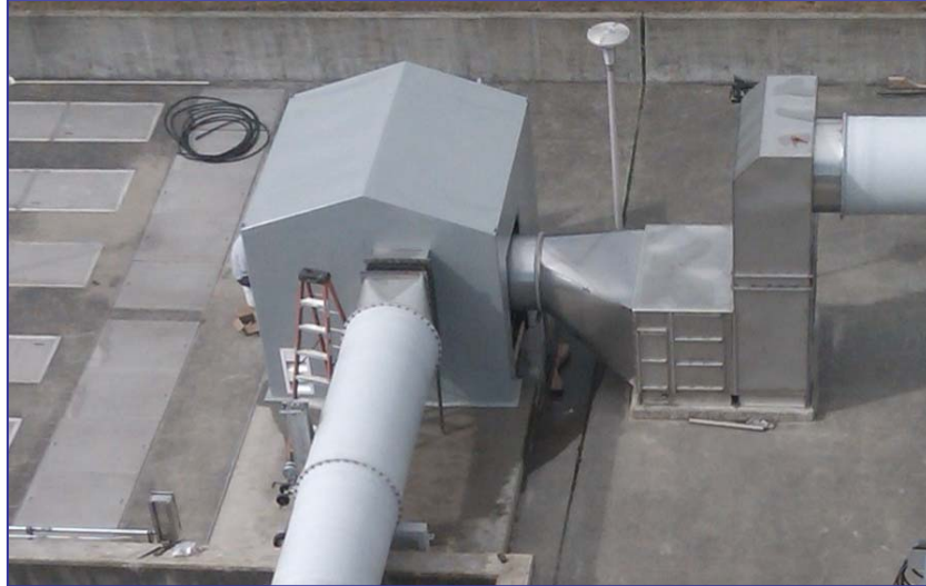
FanAir Co. 10 Ft x 10Ft x 12 FT Fiberglass Acoustic Sound Enclosure Installed at Anacortes, Washington Waste Water Treatment Plant.
