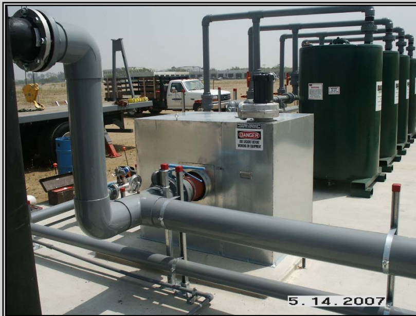
FanAir Co. 6 Ft x 6 Ft x 5 FT Fiberglass Acoustic Sound Enclosure designed and built for a Fiberglass Odor Control Blower for a Biofilter Located in Orange, County, Ca.
