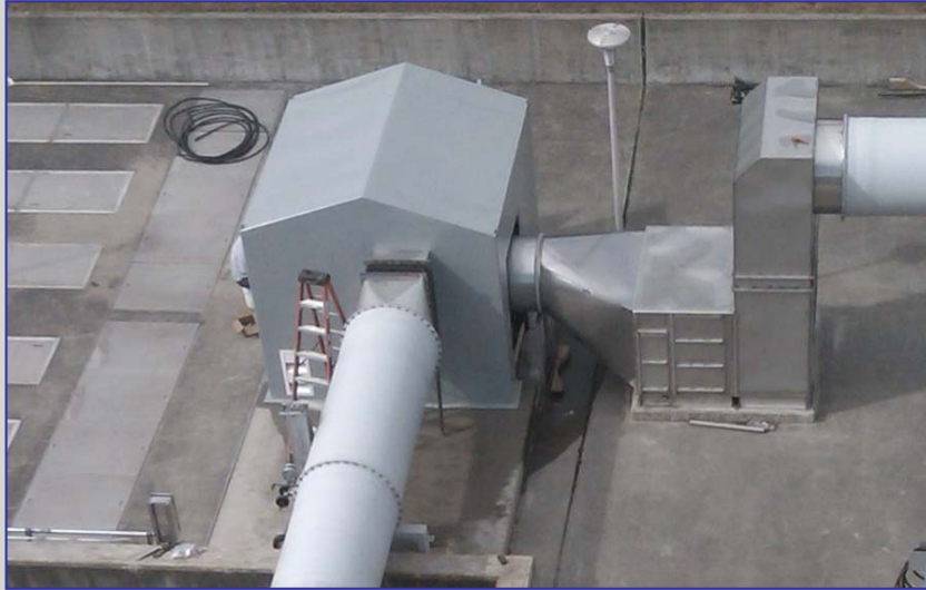
FanAir Co. 10 Ft x 10Ft x 12 FT Fiberglass Acoustic Sound Enclosure Installed at Anacortes, Washington Waste Water Treatment Plant.
