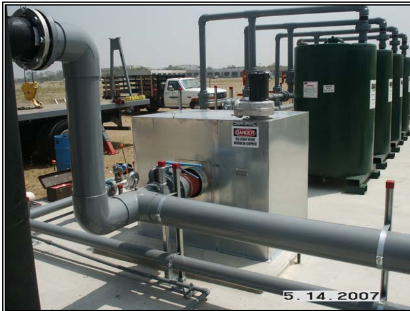
FanAir Co. 6 Ft x 6 Ft x 5 FT Fiberglass Acoustic Sound Enclosure designed and built for a Fiberglass Odor Control Blower for a Biofilter Located in Orange, County, Ca.
